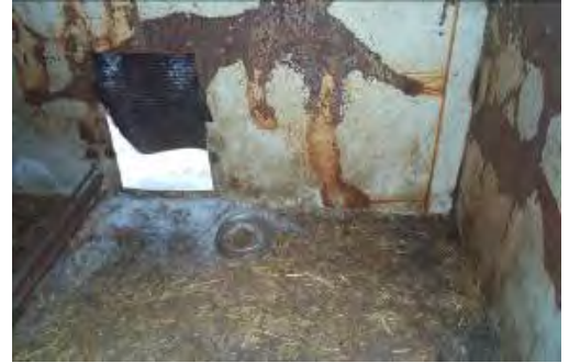
8-21. No bedding, rusted dog enclosure 3.1(c)(1)(i); 3.3(a)
